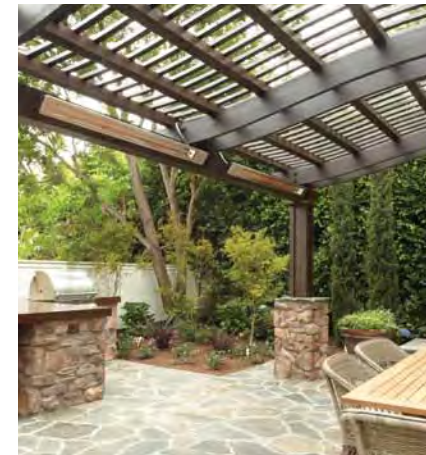
Wood pergola with Slimline heaters bracket mounted to wood beam
