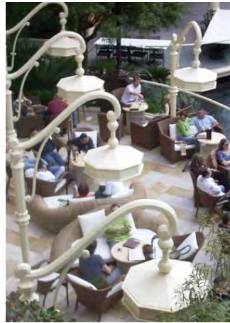
Casino patio with custom heaters, pole mounts and pendants
