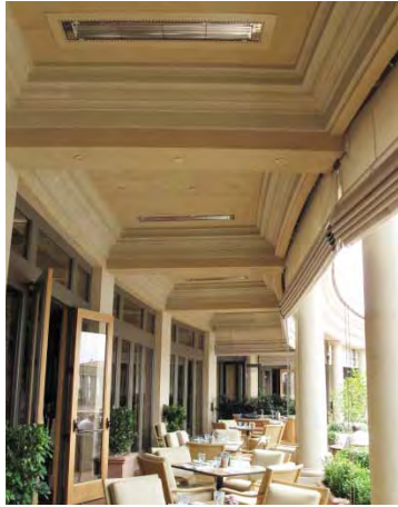
Luxury resort dining area with W-Series heaters flush mounted into a stucco coffered ceiling
