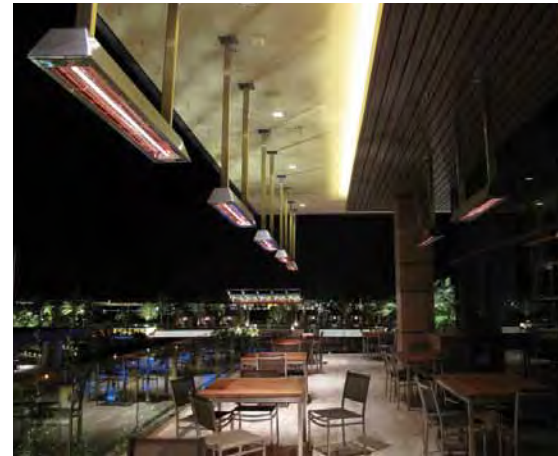
Restaurant patio with W-Series heaters ceiling mounted in custom metal shrouds
